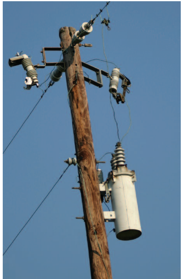
On the right of this pole, the neutral wire is missing—stolen by thieves. The replacement cost for all of their damage is estimated at more than $15,000. The crooks also left dangerous conditions, as their activity sparked a fire at the base of the pole.
