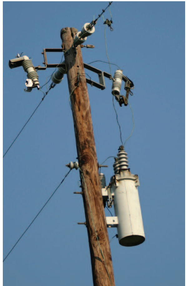
On the right of this pole, the neutral wire is missing—stolen by thieves. The replacement cost for all of their damage is estimated at more than $15,000. The crooks also left dangerous conditions, as their activity sparked a fire at the base of the pole.
